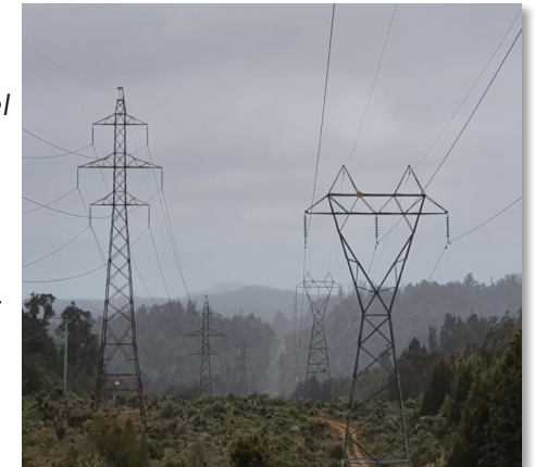
Existing transmission lines adjacent to Que River site
