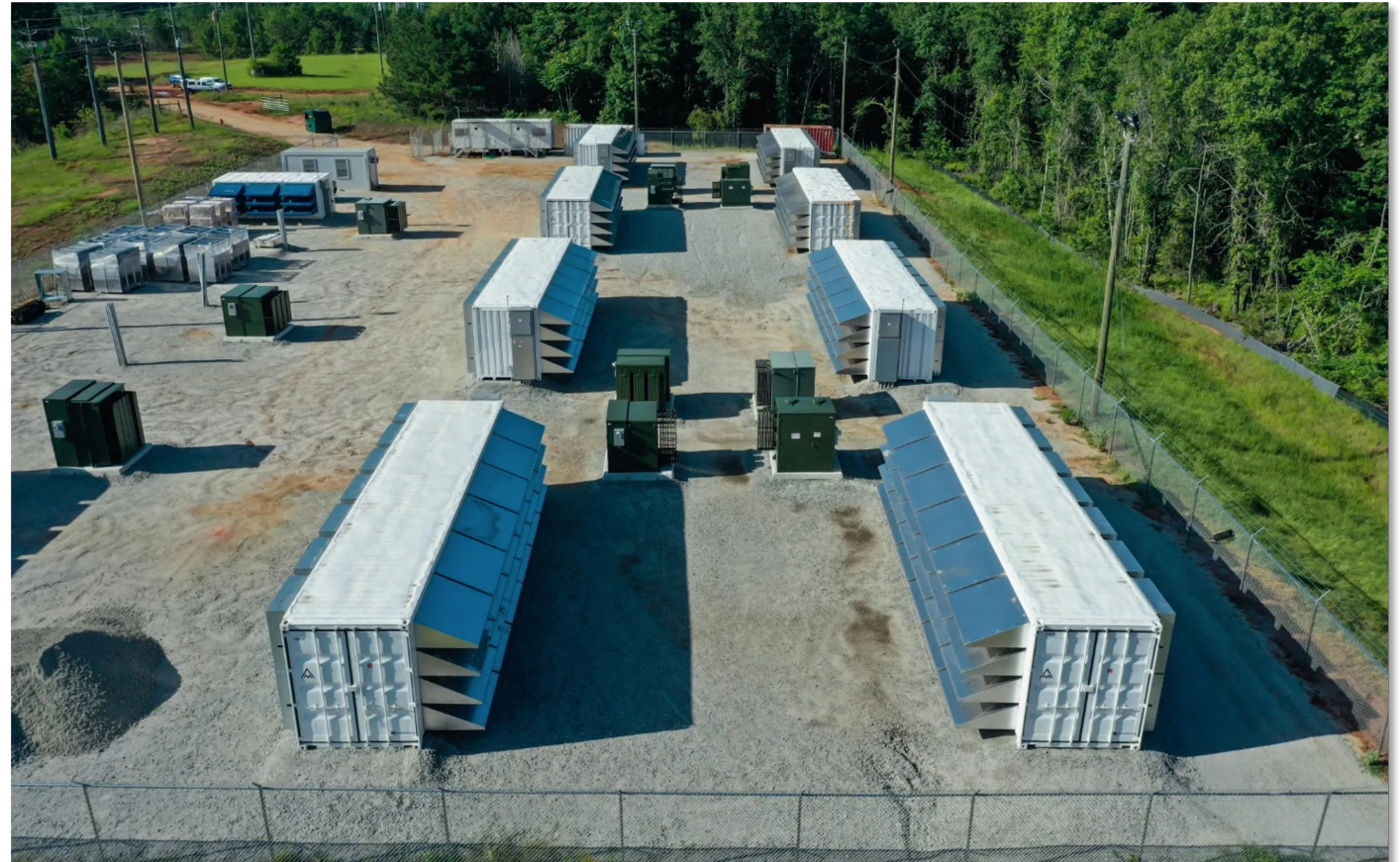
Figure: Modular Data Center Technology. Source, Mawson website
