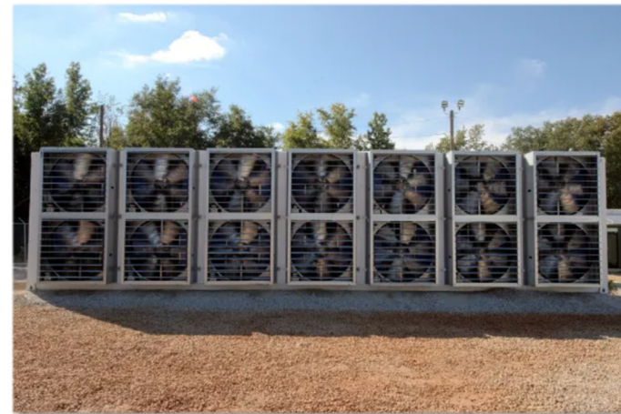
Figure: Mawson's Modular Data Centre technology
